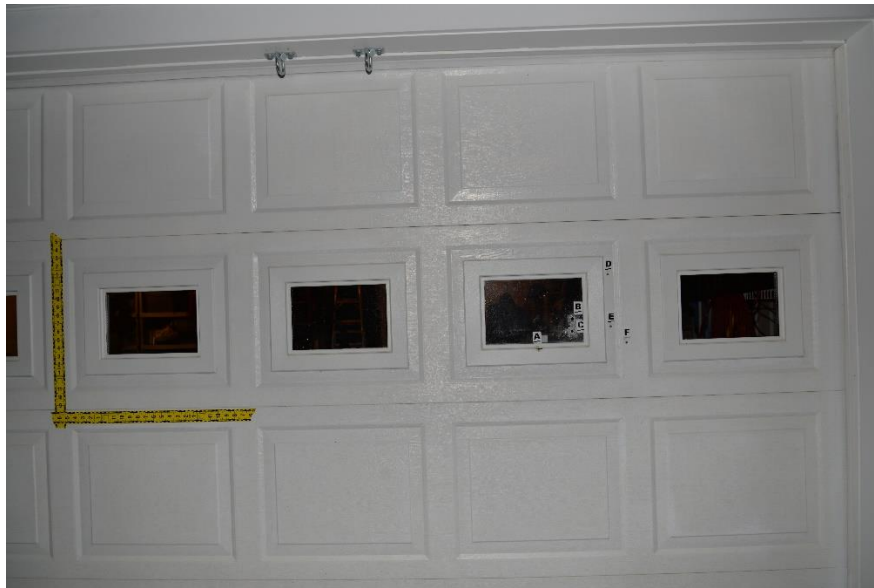
Figure 6 – Photograph showing damage to the right garage bay door.
