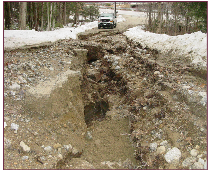
A photograph of what had been a town road, nearly obliterated by diverted runoff from the Druan property.
