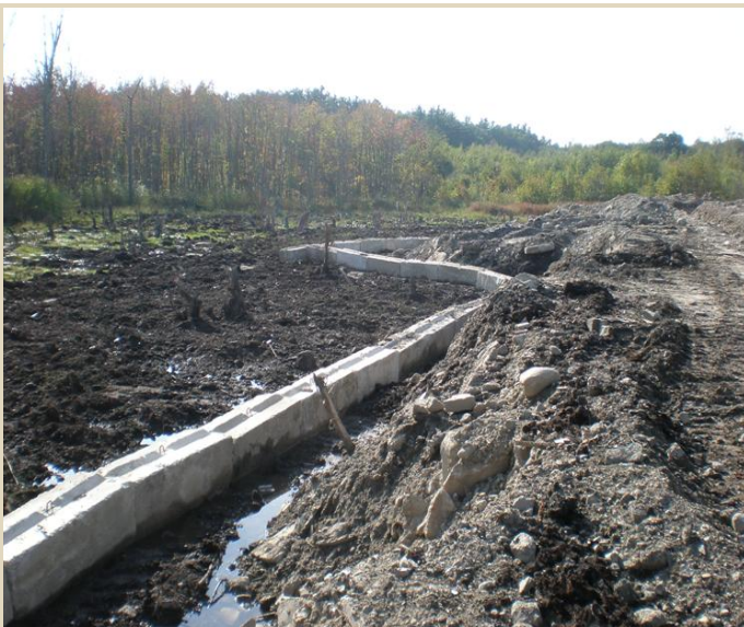
The Torrormeo Industries, Inc. wetlands restoration project in Kingston. Significant fill has been removed in the wetlands areas (left) down to the level of organic wetlands soils which will soon feature native wetlands vegetation. For years, the wetlands area had looked like the operational portion of the quarry (right), sitting under up to fifteen feet of fill. A white silt barrier divides the two areas to prevent unwanted runoff.
