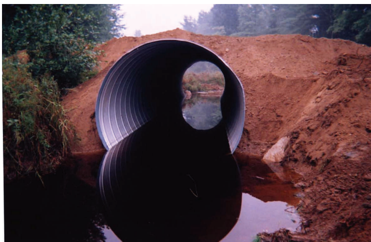
10-foot diameter culvert and destabilized soils in Bee Hole Brook, Loudon, NH.
